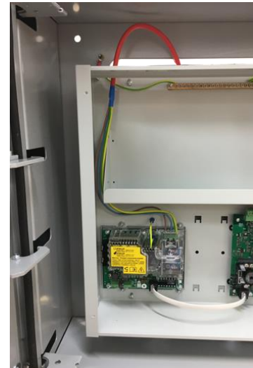
PHOTO 1 SHOWING MAINS CABLE ROUTED AND CONNECTED TO THE PSU
