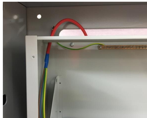
PHOTO 2: MAINS CABLES FED THROUGH TOP SLOT IN EACIE CHASSIS AND ROUTED TO PSU
