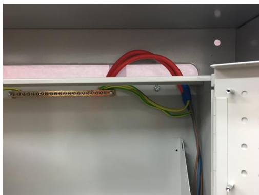
PHOTO 3: LOOP CABLES FED THROUGH TOP SLOT IN EACIE CHASSIS AND ROUTED TO MAIN CONTROL PCB
