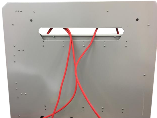
PHOTO 1: FIELD CABLES FED THROUGH REAR SLOT IN PROTECTIVE CABINET
